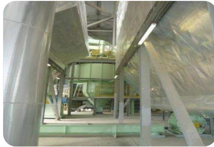
Separator with mill & process filter
