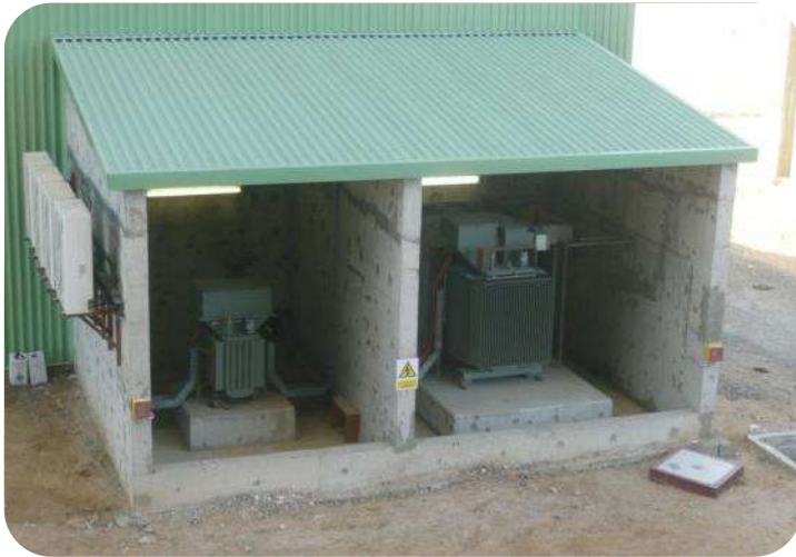
Transformer boxes for grinding plant
