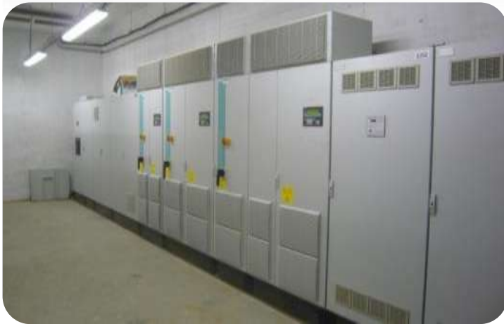
LV cabinets with frequency converters
